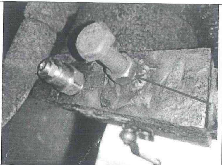
P8, The balance valve on the NO.2P and NO.7P was can not renew due to the old one had been welded on the valve block.
